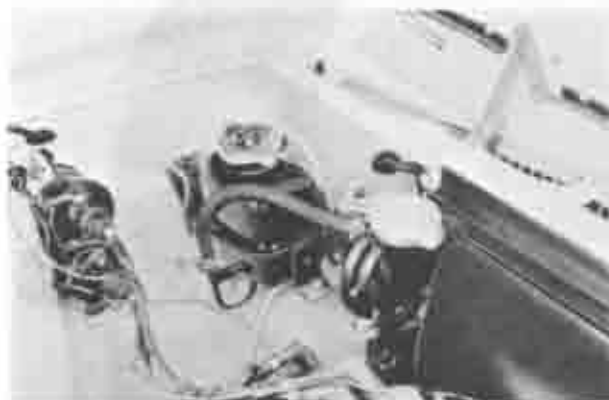
Fig. 3-2 Radiator and expansion chamber
