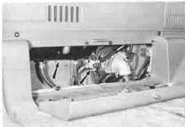
Fig. 1A-61 Condense tank and check valve (Wagon)
